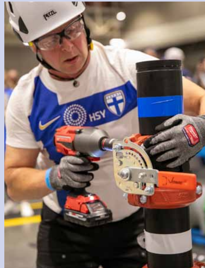
This year’s Collection Systems Event tasked teams with assembling a Victaulic (Easton, Pennsylvania) pipe tower rather than programming an autosampler, as in past competitions. Many participants praised this substitution despite reporting difficulties in adapting their approaches to the event. Kieffer Photography
