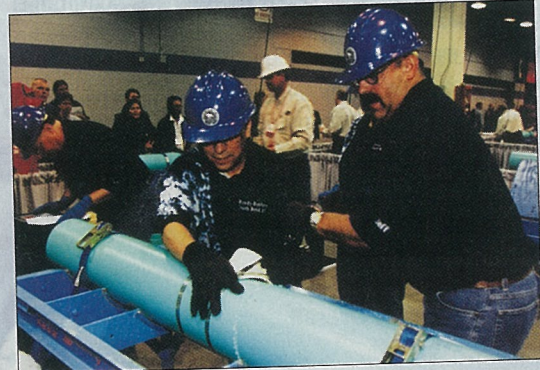
Indiana's Richmond Rotifers repair an in-service section of pipe in the collections event.
