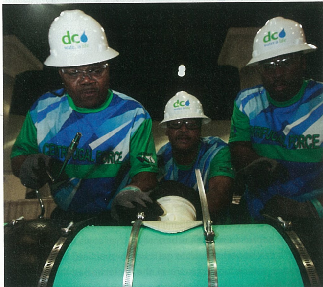
Moses Riley, Melvin Keys, and Aaron Montgomery, Centrifugal Force team members from the Chesapeake Water Environment Association, work to attach the service saddle on the replacement pipe. This year, in addition to the pipe repair, teams had to identify six pipe defects in a quiz. Kieffer Photography
